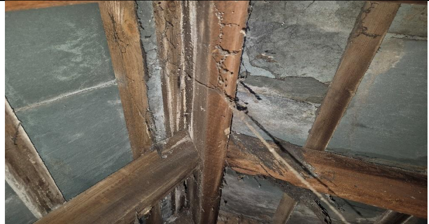
Figure 26 - Delaminating slates at ridge
