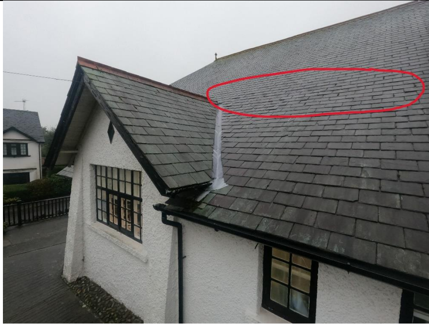
Figure 7 - Large area of loose and unstable slate
