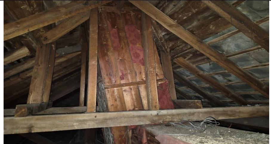
Figure 30 - Wall paper on air box vent
