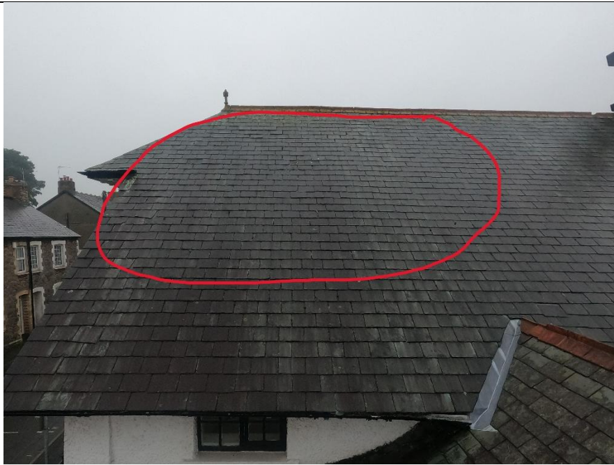
Figure 5 – Large loose area of slate
