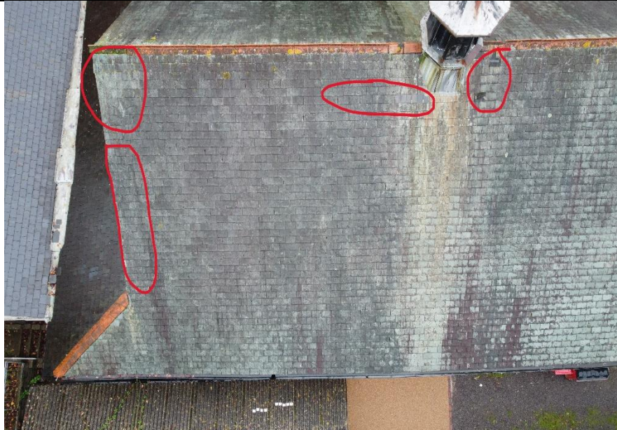
Figure 13 - Loose and/or broken slate
