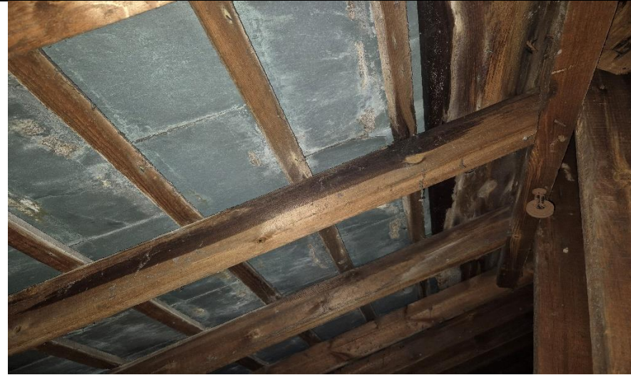
Figure 34 - Water ingress below vent box
