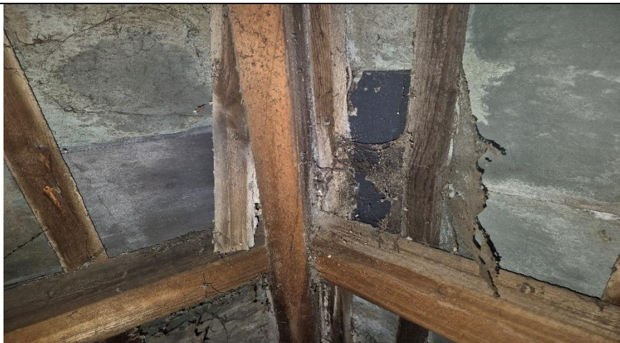
Figure 31 - Slate delamination & timber rot at ridge
