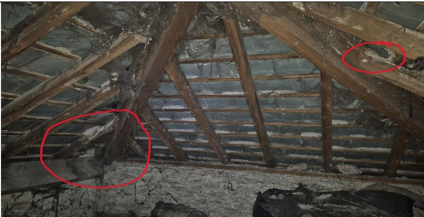
Figure 27 - Water ingress at hip (See fig 12)
