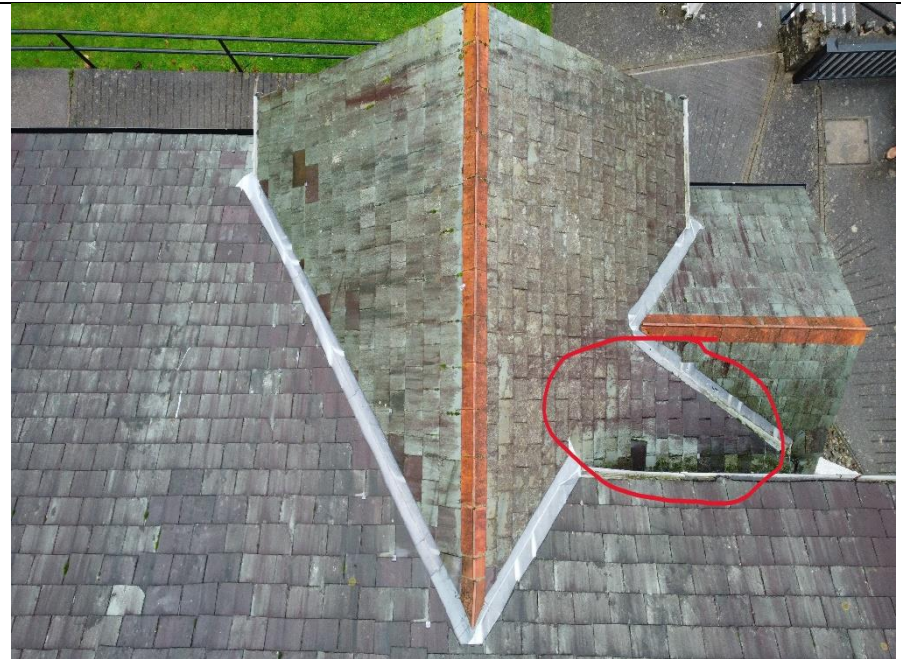
Figure 6 - Loose and broken slate
