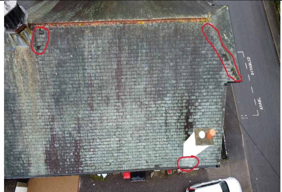
Figure 14 - Slipped and/or broken slate
