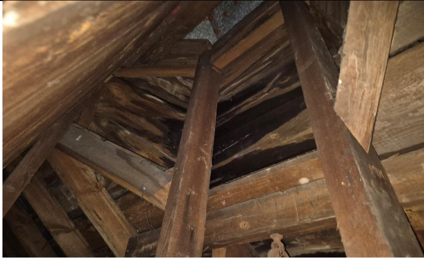
Figure 33 - Water ingress to west side of vent box
